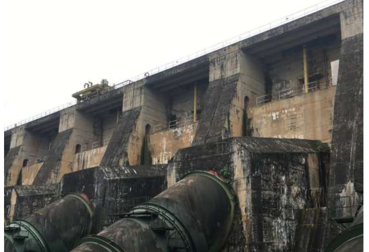
Cracked Concrete Siding
